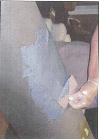
The defect must be completely filled in and the compound must be smoothed and leveled out. Remove high spots and fill any low spots.
