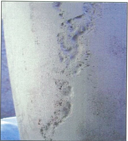
Fig. 1 – The sandblasting done on this line revealed more damage than was visible during the initial inspection. Proper cleaning is essential to a sound repair.
